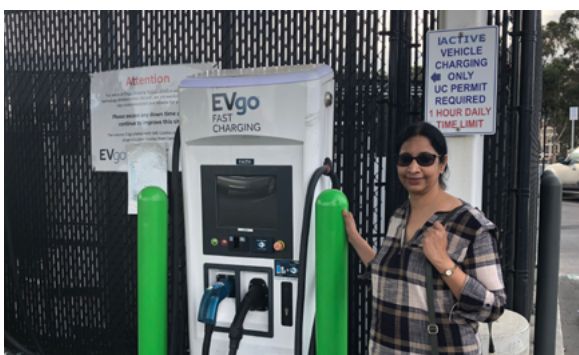
PLF Aruna Sundararajan toured UC San Diego's electric vehicle charging infrastructure initiative.
